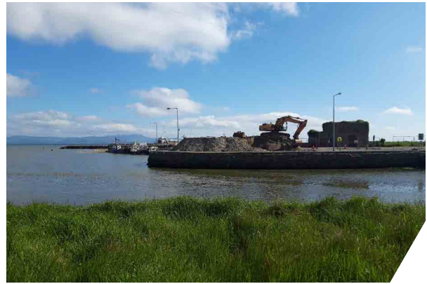
Dredging works in Annagassan – in 2021 dredging works were carried out at the harbour in Annagassan
