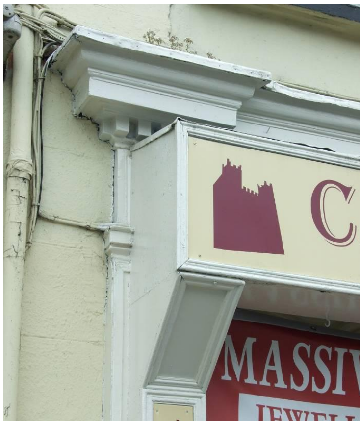
Fig. 127: Inappropriate alterations obscuring a decorative shopfront
