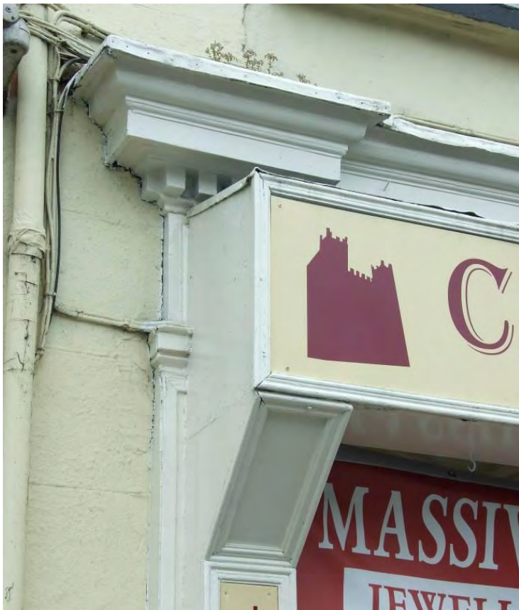
Fig. 127: Inappropriate alterations obscuring a decorative shopfront
