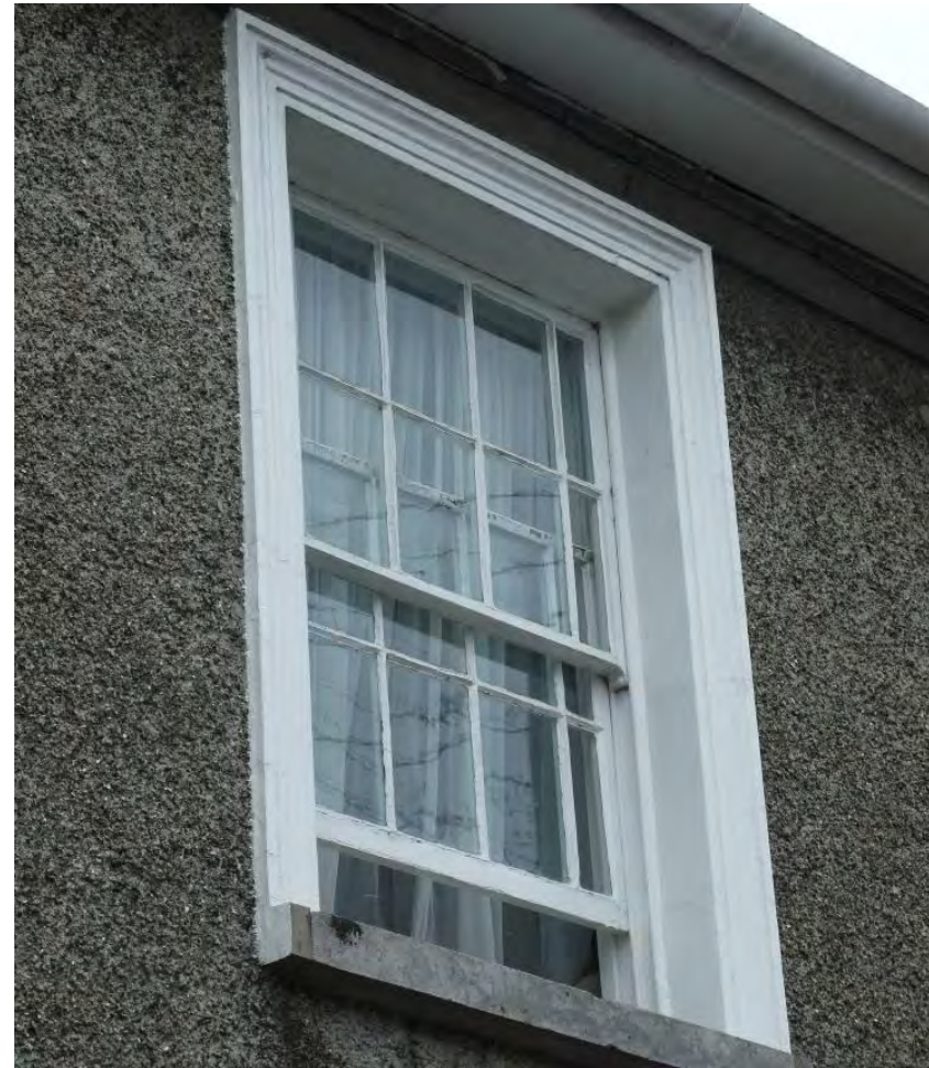
Fig. 117: Historic windows are perhaps the single most important element of an historic streetscape
