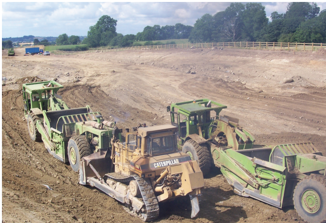
Major earthworks underway at Thistle Cross on the A1/N1 Newry Dundalk Link Road.
